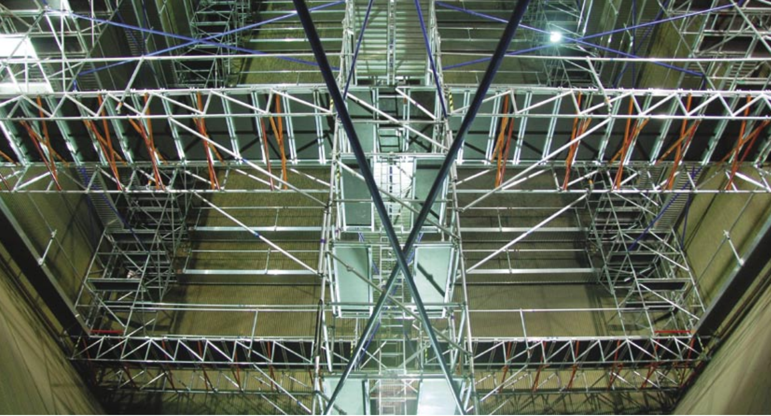
Above: Manjung Boiler Access System, Malaysia 660MW unit commissioned in November 2007. View looking from the bottom of the hopper showing base trusses and upper structure.
